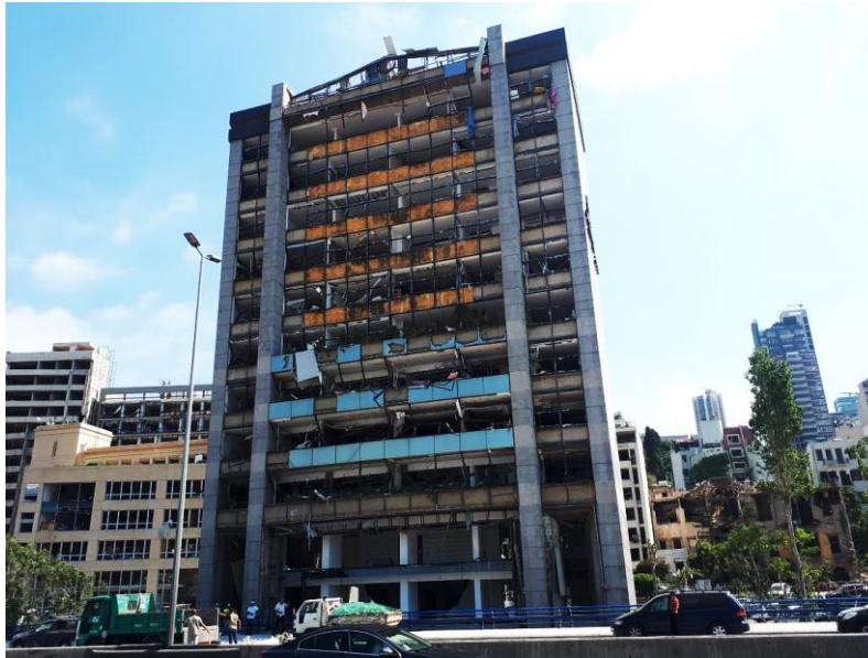
Figure 2: structural damages to buildings after the Beirut port explosion (credit: dpa/picture alliance)
